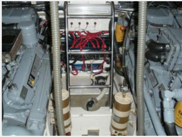
Very Clean Engine Room
