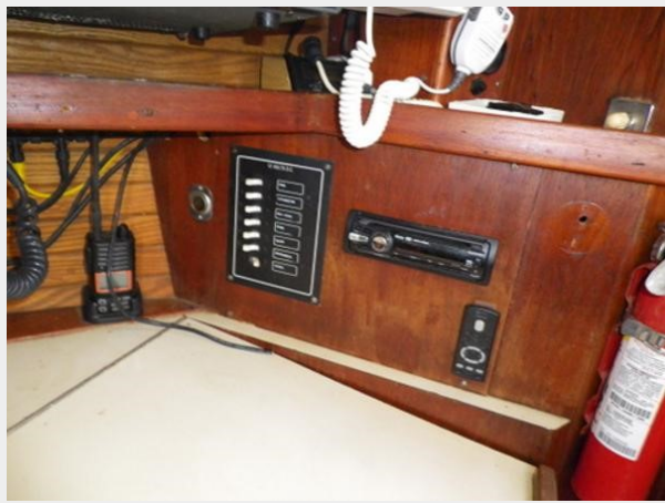
Power Panel at Nav Station
