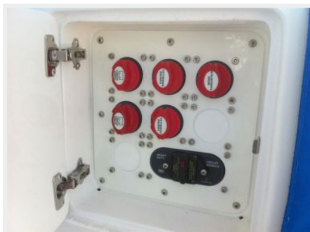
Battery selector switches
