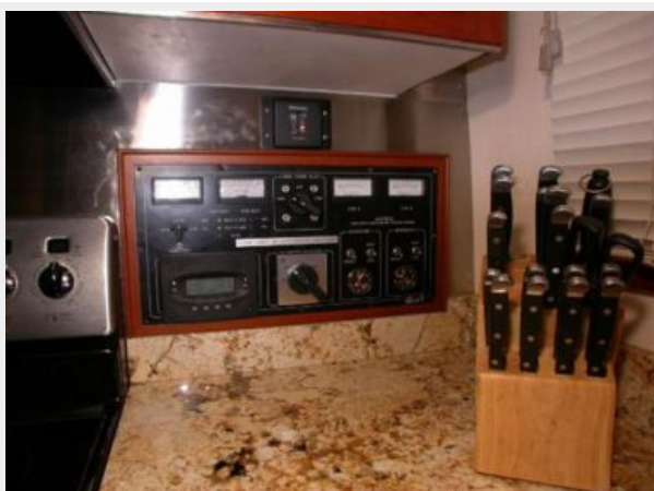
Galley Elect Load Center
