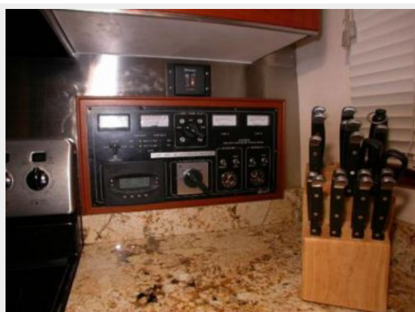
Galley Elect Load Center
