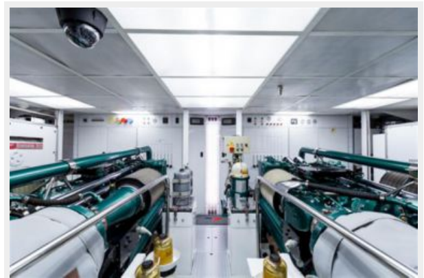
Engine Room Forward View
