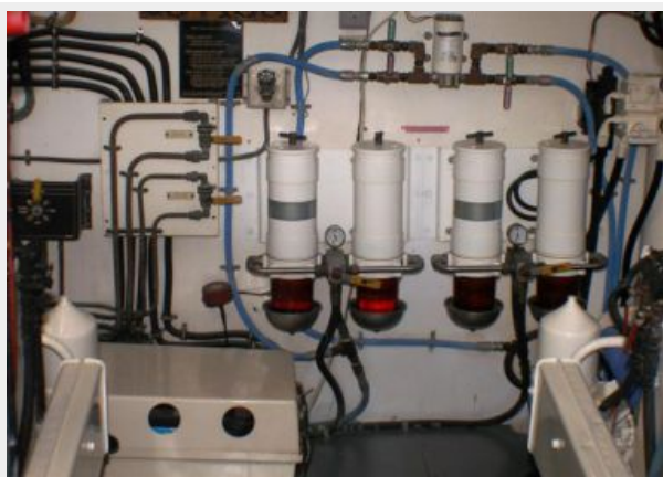
Engine Room - Fuel Filtration
