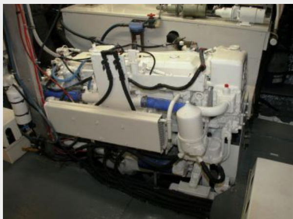
Engine Room - Port Side
