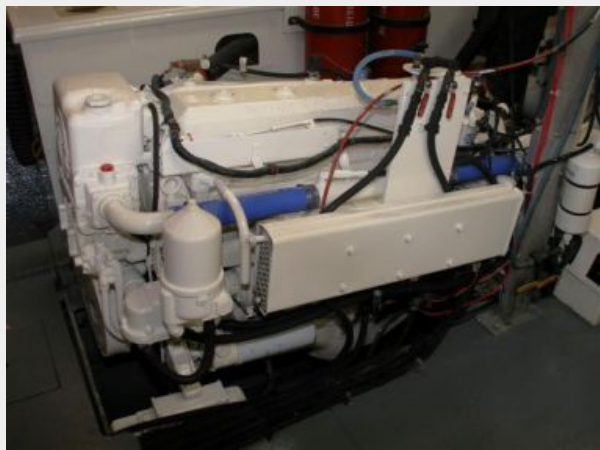
Engine Room - Stbd
