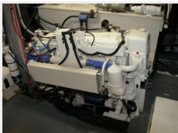
Engine Room - Port Side
