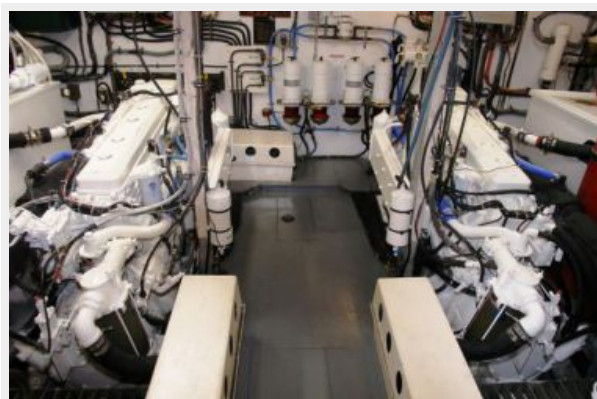
Engine Room - View Fwd
