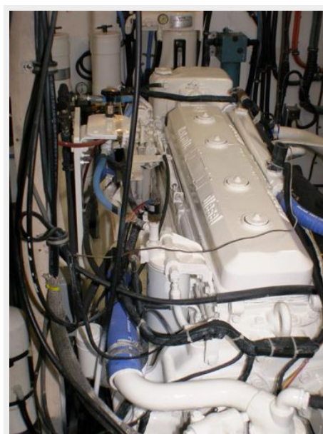
Engine Room - Port Main
