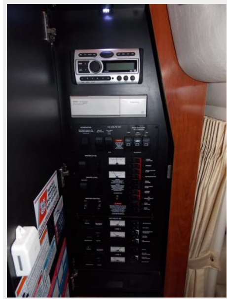
Main Distribution Panel
