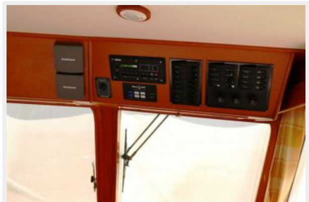
Lower Helm Overhead
