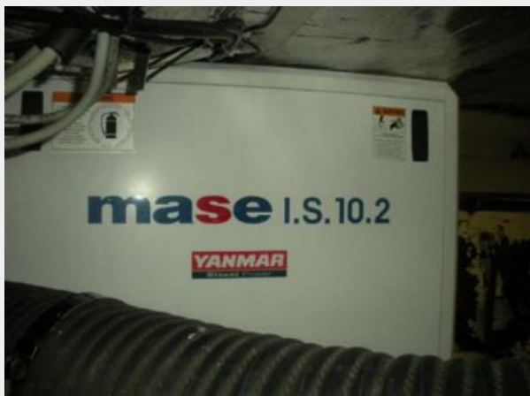
New Mase Generator - 10 Hours
