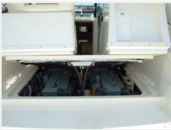
Helm Deck Lift
