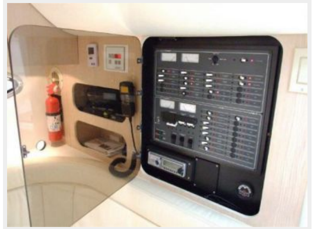
Electrical Panel Salon
