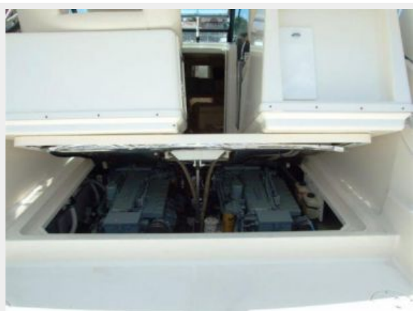
Helm Deck Lift
