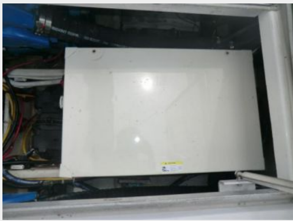
Generator with Cover
