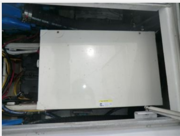
Generator with Cover
