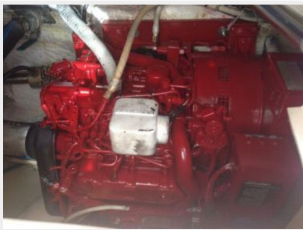
Engine & Mechanical Equipment 2
