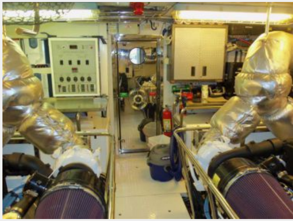
Engine Room Looking Aft
