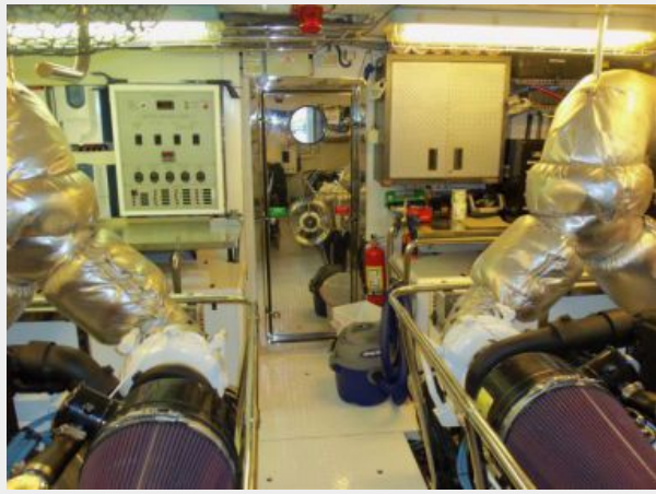
Engine Room Looking Aft
