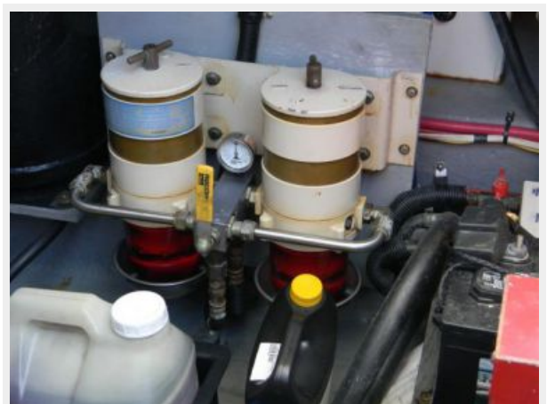
Racor Filters - Starboard
