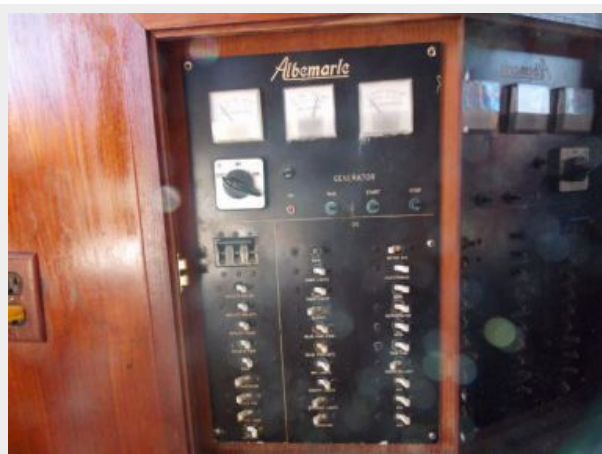
325 Albemarle, breaker panel
