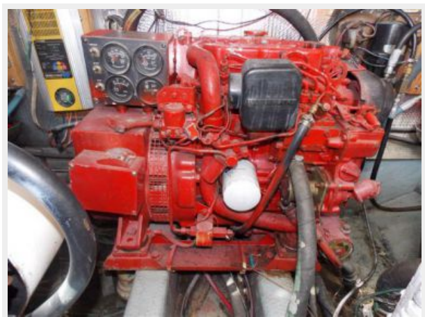
325 Albemarle, diesel generator
