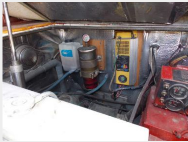
325 Albemarle, battery charger
