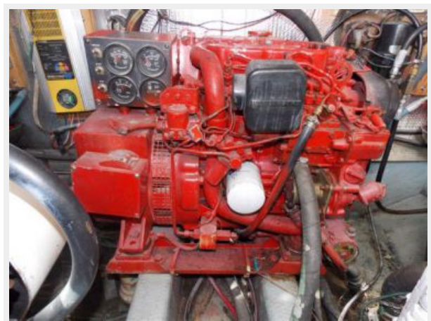
325 Albemarle, diesel generator
