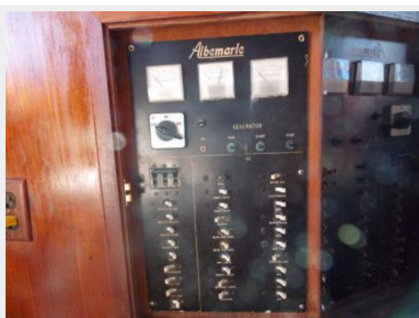
325 Albemarle, breaker panel
