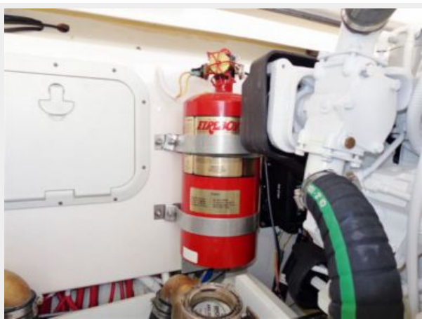
Fire Suppression System
