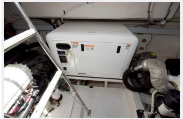
Engine Room- Generator
