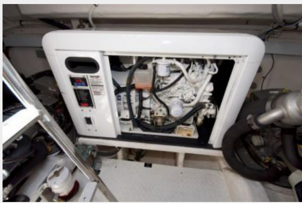
Engine Room- Generator
