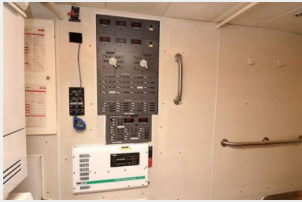
Engine Room Controls
