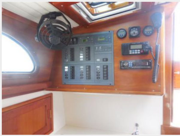
Panels and Controls
