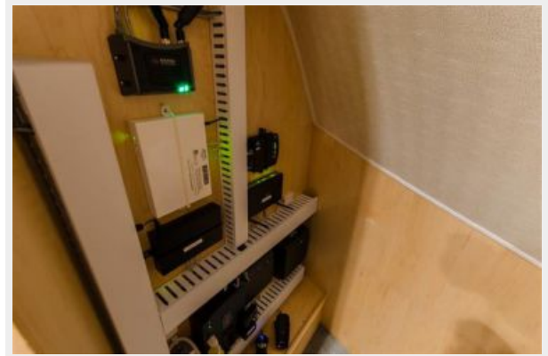
Electrical Storage Area
