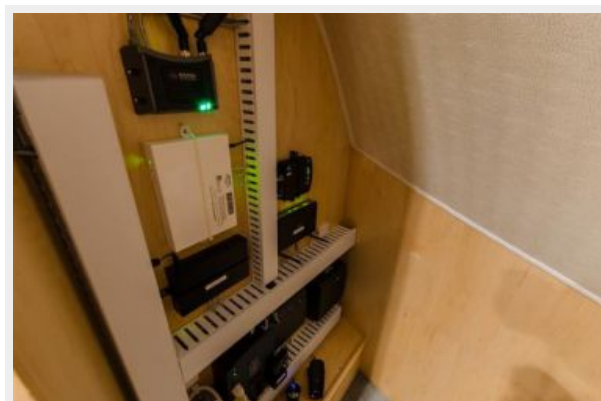
Electrical Storage Area
