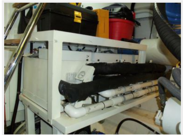
Chilled Water AC
