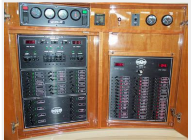
Main Electrical Panel
