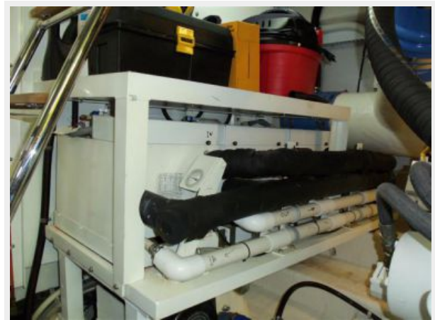
Chilled Water AC
