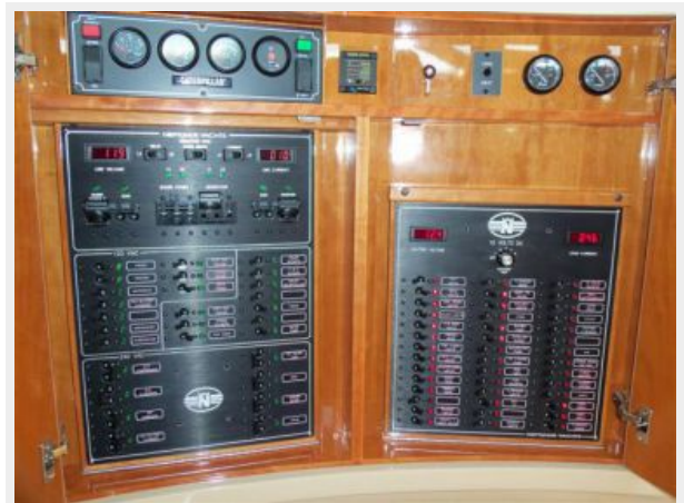
Main Electrical Panel
