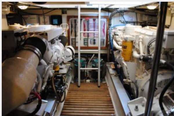
Engine Room Looking Forward
