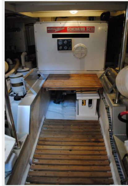
Engine Room Looking Aft
