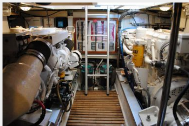
Engine Room Looking Forward
