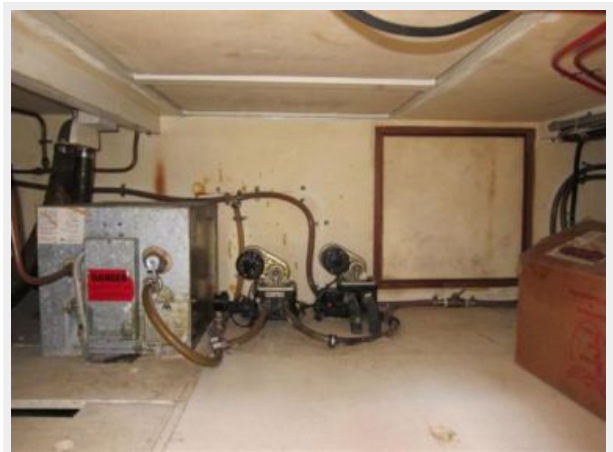
Midship storage engine compartment
