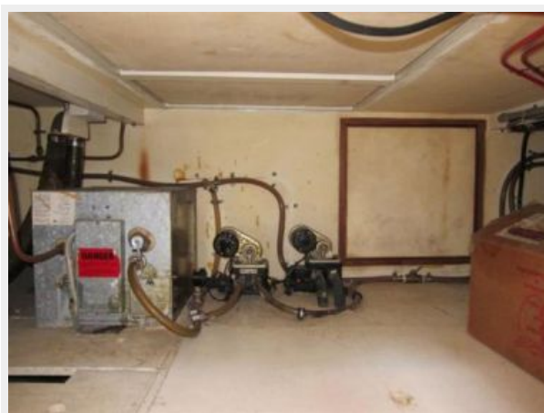
Midship storage engine compartment
