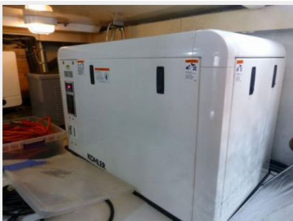
One of the two 2012 new Gensets (Both 120 hours)
