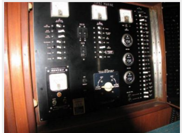
Electrical System 1 - Electrical Panel
