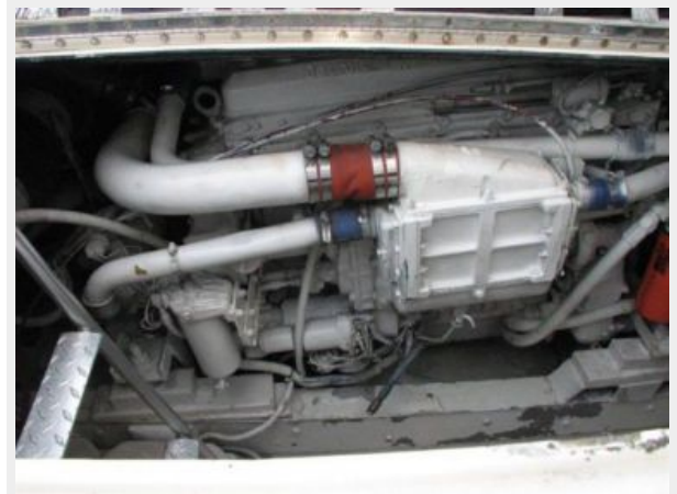
Engine & Mechanical Equipment 2 - Port Engine
