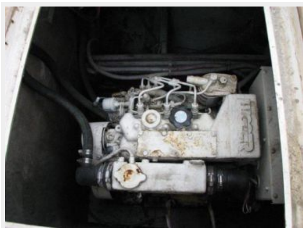
Electrical System 2 - Generator
