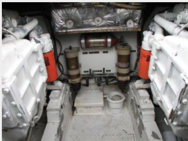
Engine & Mechanical Equipment 1 - Engine Room
