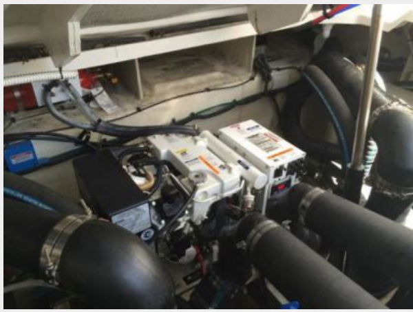
Kohler 5kW Generator
