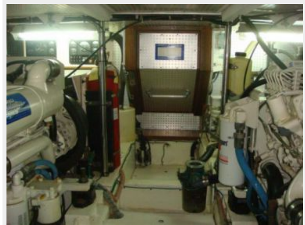
48' Novatec engine room forward
