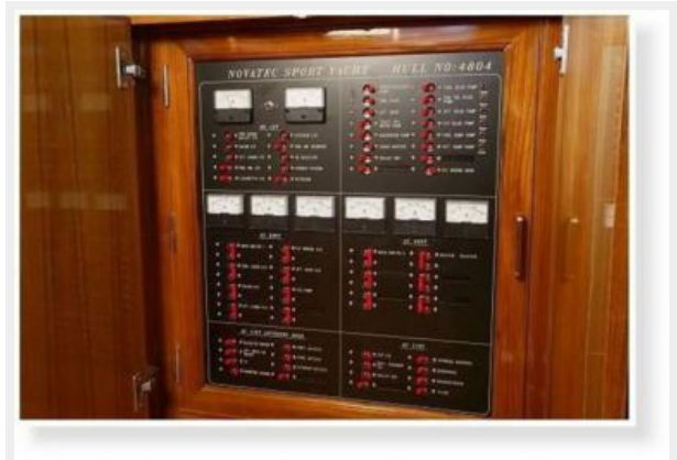
48' Novatec electrical panel
