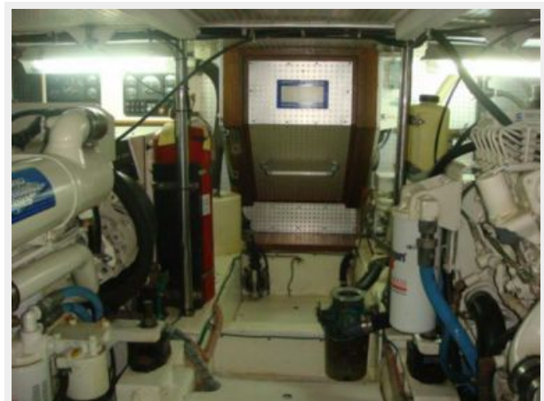
48' Novatec engine room forward
