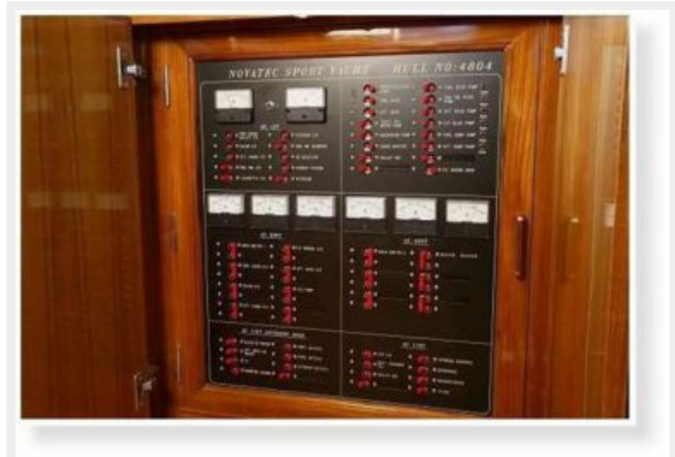
48' Novatec electrical panel
