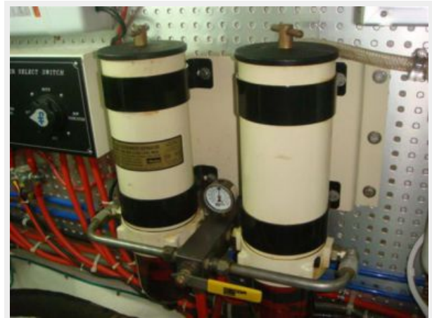
48' Novatec starboard Racor fuel filters
