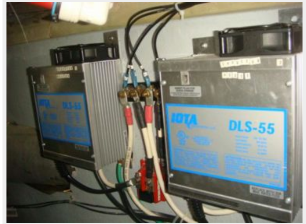
32' Levy battery chargers
