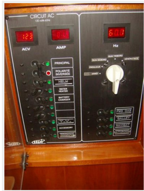
32' Levy electrical panel2
