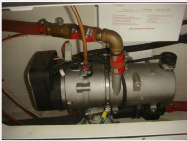
32' Levy heating system
