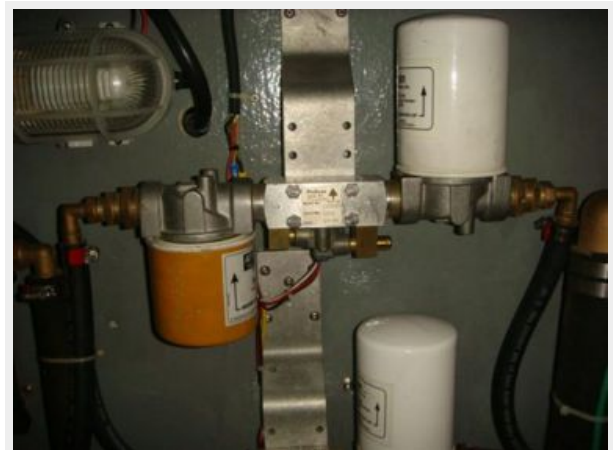
32' Levy FloScan fuel monitoring system
