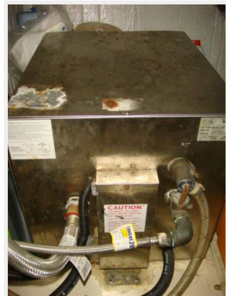
34' American Tug water heater
