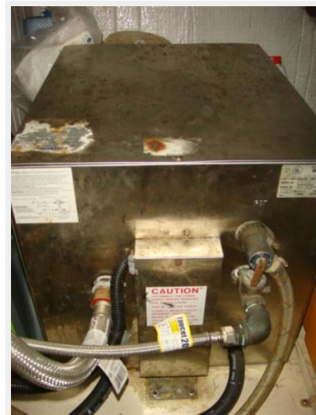
34' American Tug water heater
