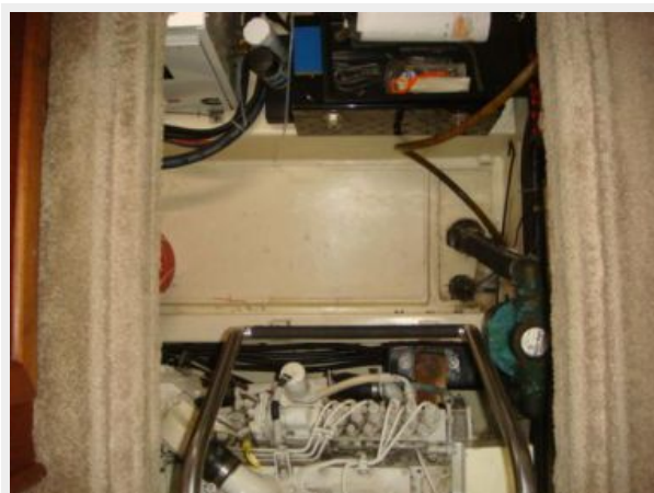
34' American Tug engine room port access
