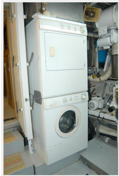
Engine Room Washer & Dryer
