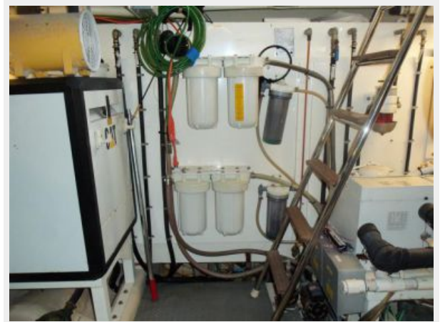
Engine Room Aft
