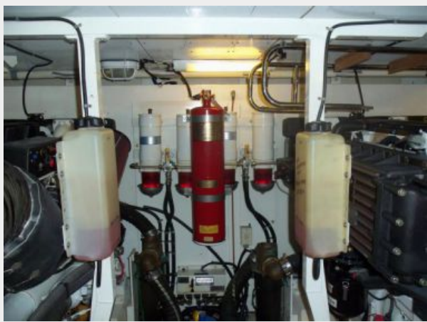
Engine Room Forward
