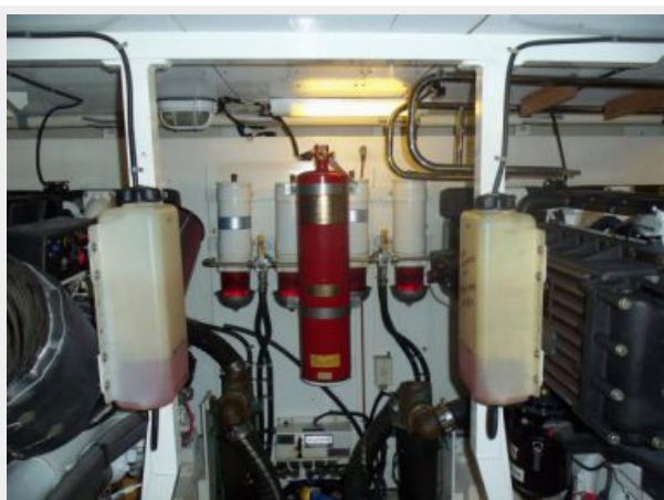
Engine Room Forward
