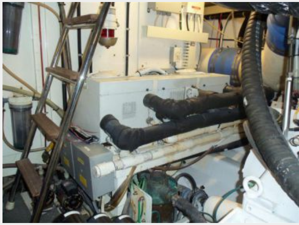
Chilled Water AC
