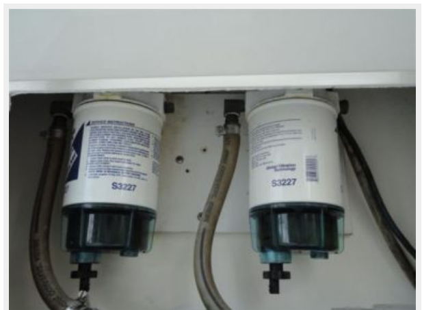
Engine Fuel Pumps
