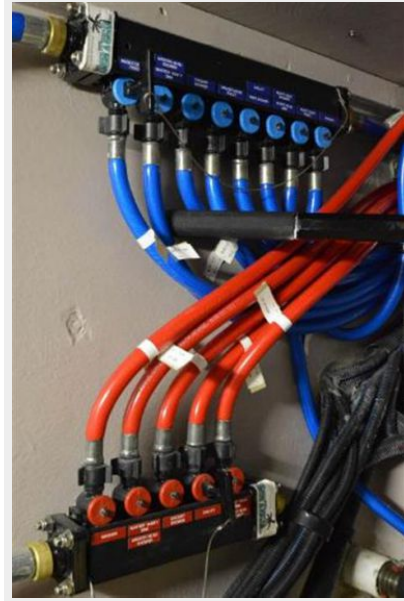
Fresh Manifold in Utility Room
