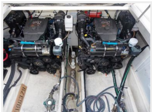
Engine Room w/ Fresh Water Flush
