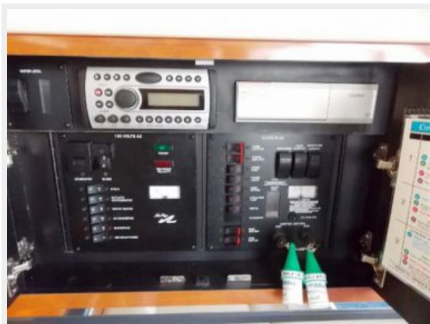
Main Distribution Panel
