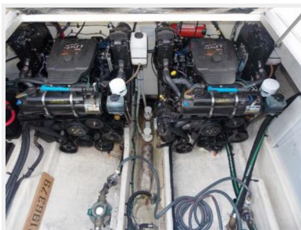
Engine Room w/ Fresh Water Flush
