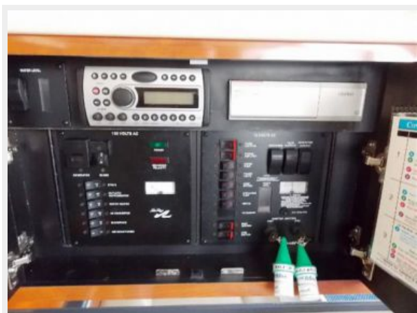
Main Distribution Panel
