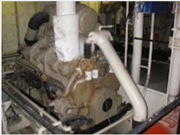
75 KW - Auxilliary Generator
