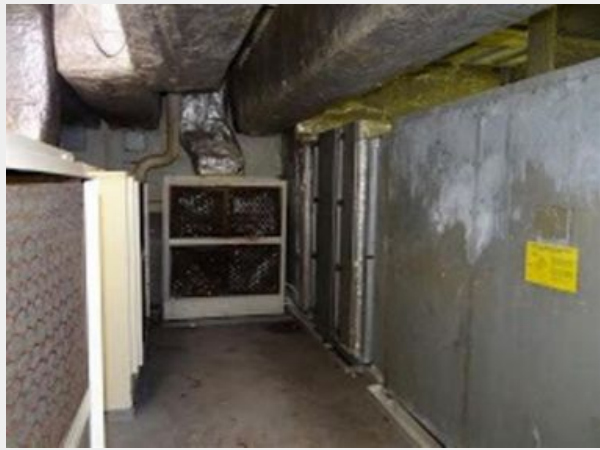
Air Conditioning - Filter Room
