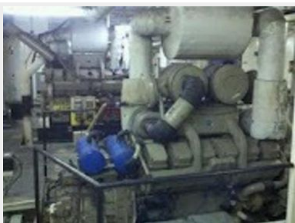
CAT - T-38 - MAIN ENGINES
