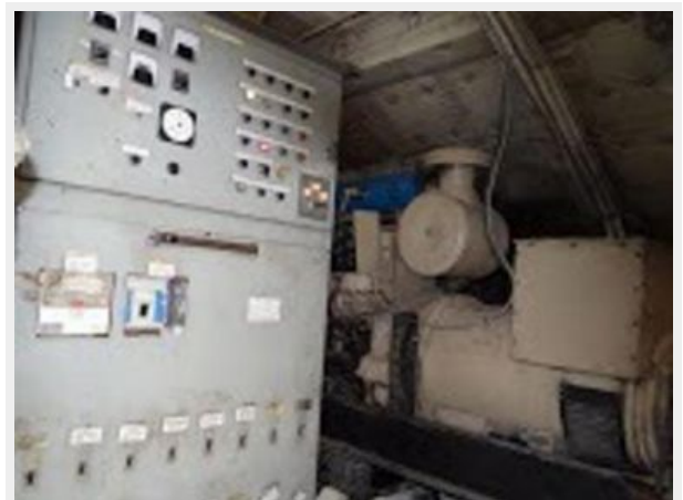
Generator Switch Panel
