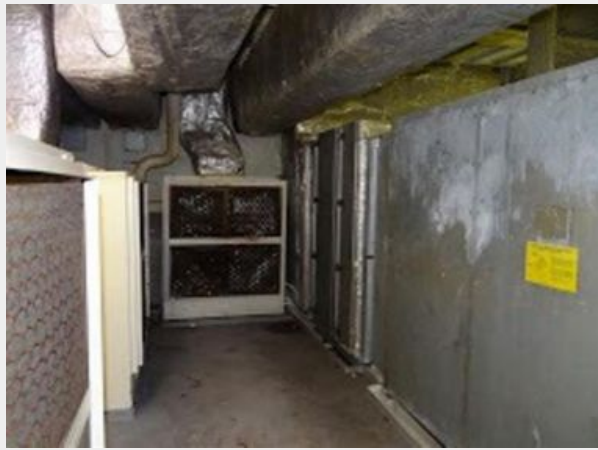
Air Conditioning - Filter Room
