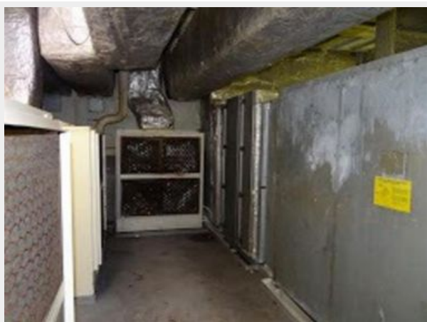
Air Conditioning Space
