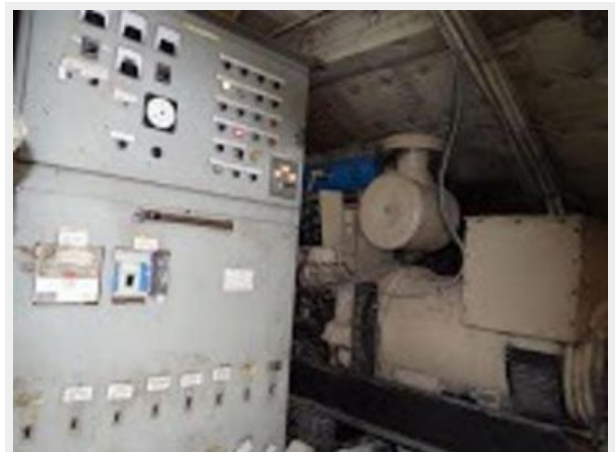
Generator Switch Panel
