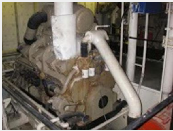
75 KW - Auxilliary Generator
